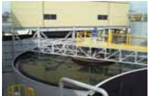
Turbid water treatment
