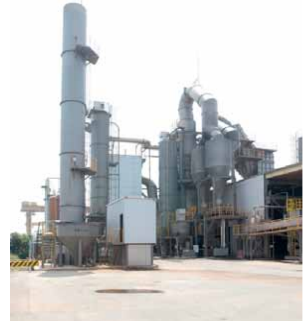
Exhaust Gas Treatment Facilities
