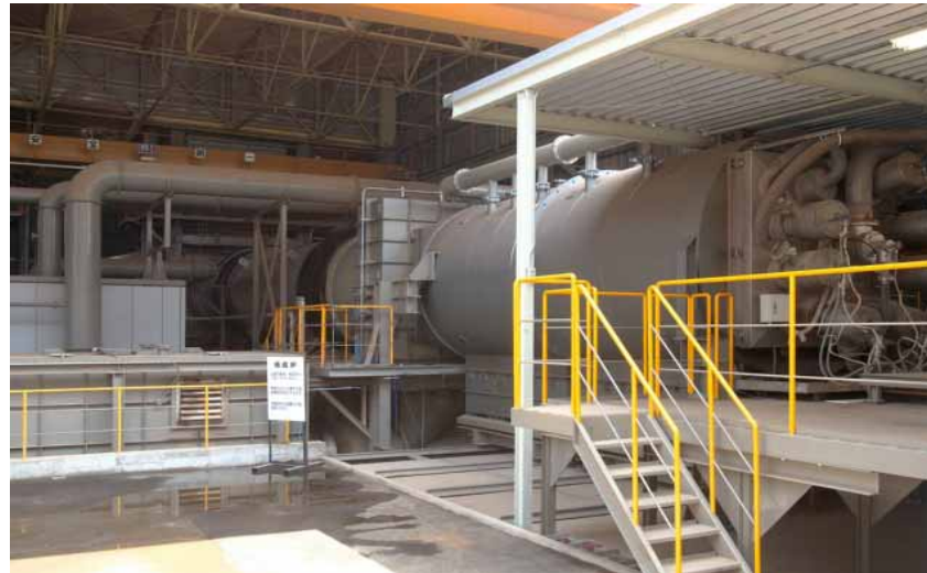
Heating Furnace of Handa Plant
